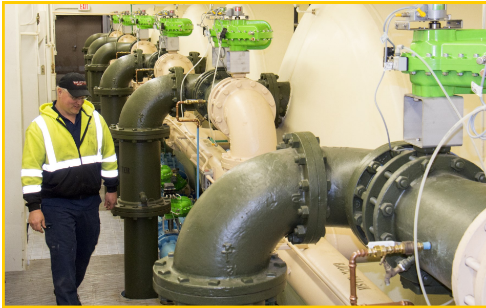
Keeping your drinking water safe at Commons Park Filtration Plant.
