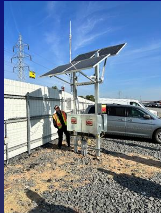
Figure 1: A Fridley staff member views the solar-powered battery for the electric fence at 3737 East River Road during a site visit on September 14, 2023. The existing fence and corrugated metal barrier are visible in the background.
